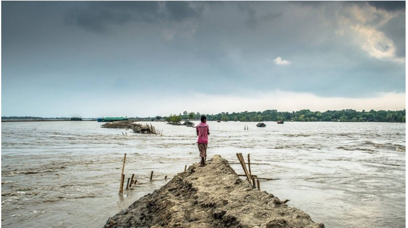
Photo 11.1 The third breach in the realigned embankment (August 2015)
