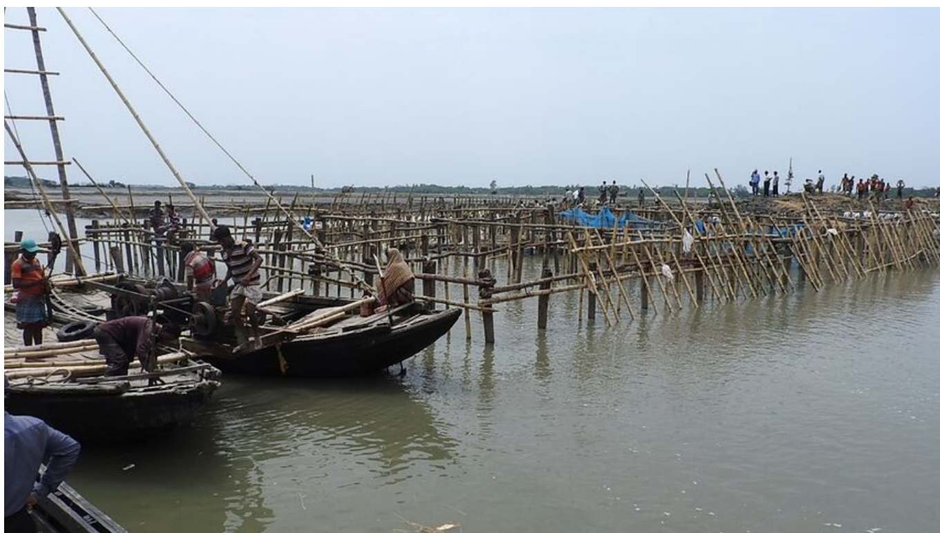
Photo 11.3 Driving bullah piles in Breach 3 to provide a framework for sand-filled geobags
